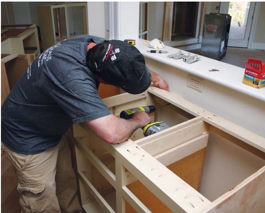
Figure 11. Here, the author blocks a backless drawer base off the wall to increase countertop depth, using structural star-drive screws to fasten it to the wall framing.
