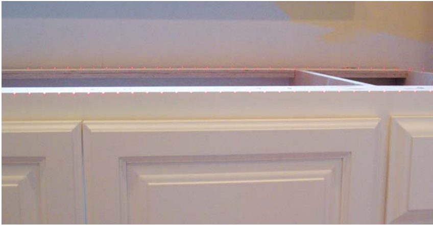
Figure 10. Splitting the laser dots between the front edge of the cabinet and the wall line provides a level reference side to side and front to back. This ensures dead-true support for a stone countertop and eliminates unsightly shim gaps.
