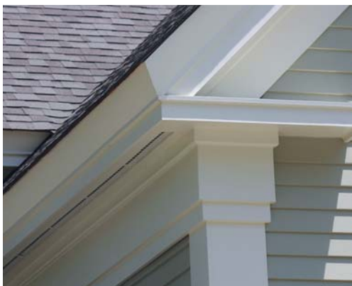
Figure 2. Considering its age, this mid-19th-century Greek Revival cornice (far left) has held up well. Note the split fillet where the rake crown molding resolves into the profiled wood gutter along the eaves. At left, the author’s modern interpretation.
