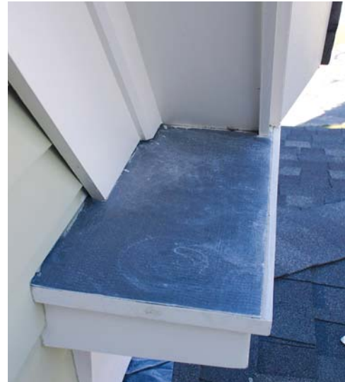
Figure 7. The eaves frieze wraps the corner and works in conjunction with the cornice to create the illusion of a capital over the corner board “column” (above left). Lead flashing caps the cornice, and the rake frieze dies on top (above).
